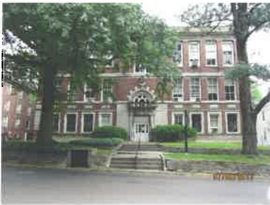
Before: Windows needed replaced at Tupper Hall
